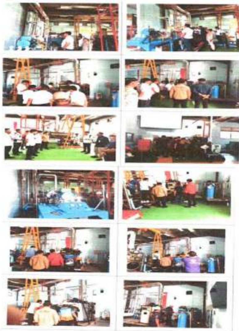
Gambar 4. 11 Pengadaan Steam Boiler
